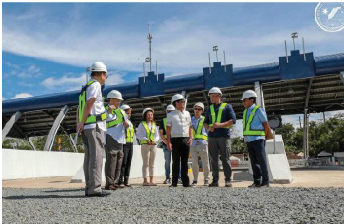
EASING CONGESTION. President Ferdinand R. Marcos Jr. inspects the ongoing construction of the Cavite-Laguna Expressway (CALAX) Governor's Drive Interchange in General Trias, Cavite, on Friday (March 21, 2025). The project, currently 44 percent complete, aims to ease traffic congestion and improve connectivity between key economic hubs. (Photo from PCO)
